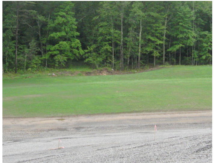
Former Chemical Pit Area Looking East Liner and Backfill Placed then Hydro-Seeded
